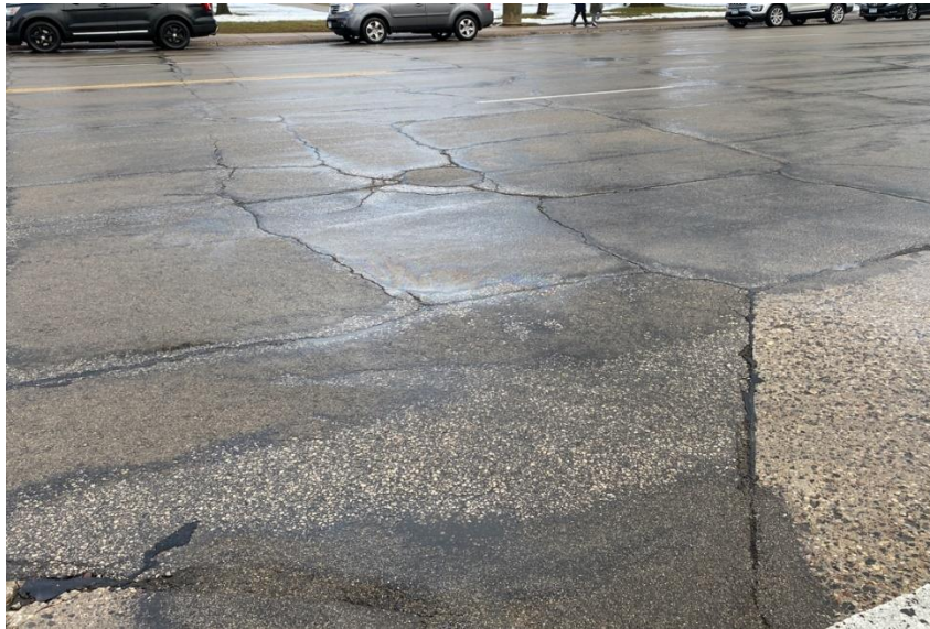
Figure 2-4 – Intersection of Cedar Ave and Main St – Cracking
