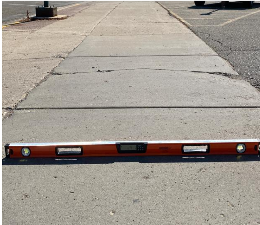
Figure 2-10 – South Sidewalk East of Oak Ave – Deteriorated, Cracked and 2.9% slope.
