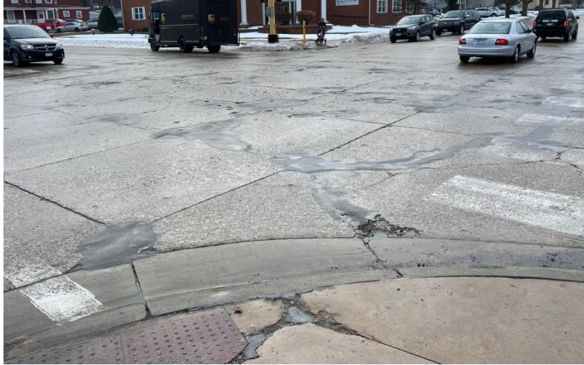
Figure 2-3 – Intersection of Elm Ave and Main St – Shows cracking and previous patching.
